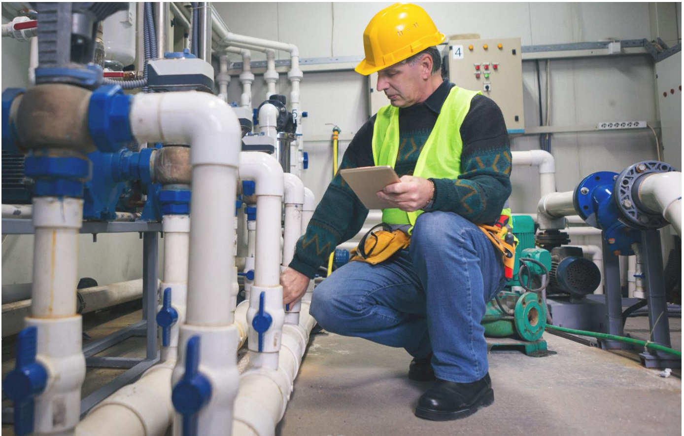
Figure 11: Regular maintenance can reduce the risk of pollution by preventing spills and leaks before they happen.
