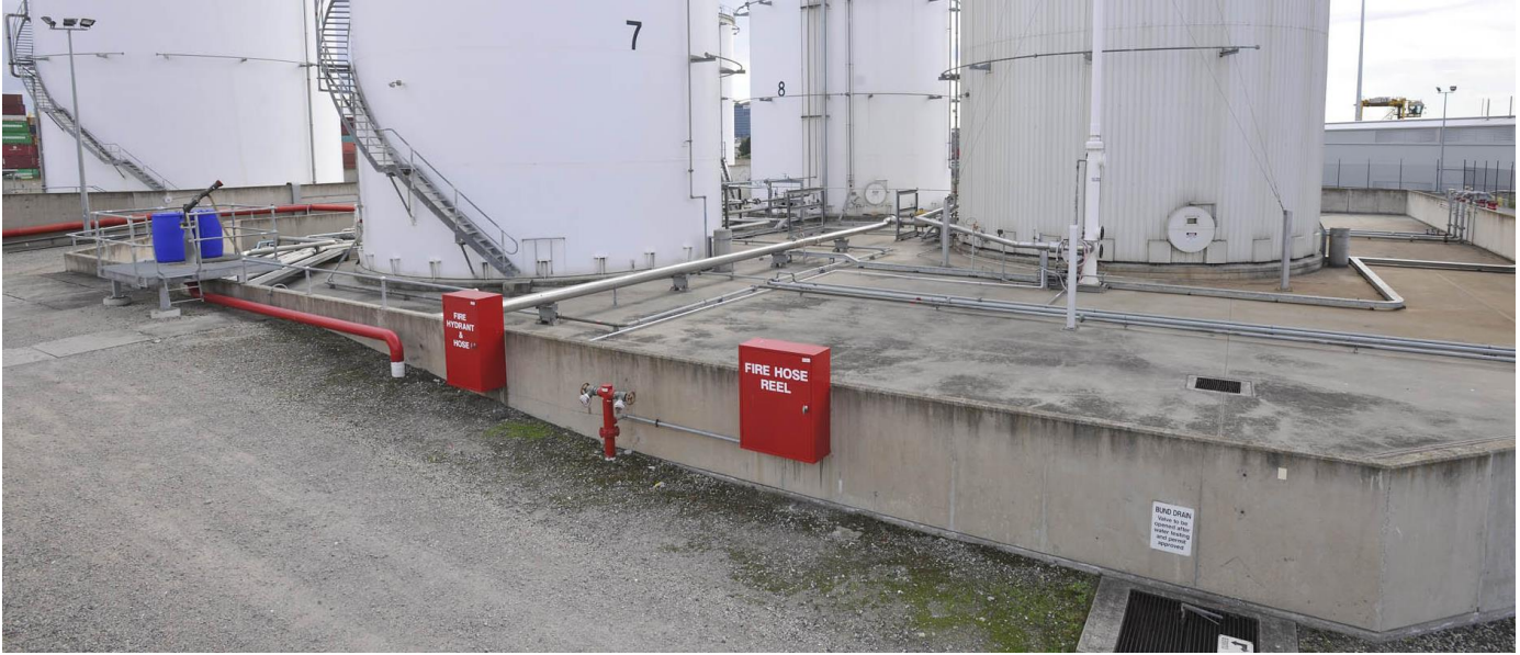
Figure 5: Image of an industry site that uses bunding around their tanks as secondary containment.
