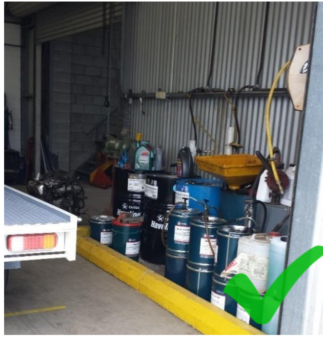
Good practice: Liquid containers stored undercover in a clearly designated secondary containment area.
