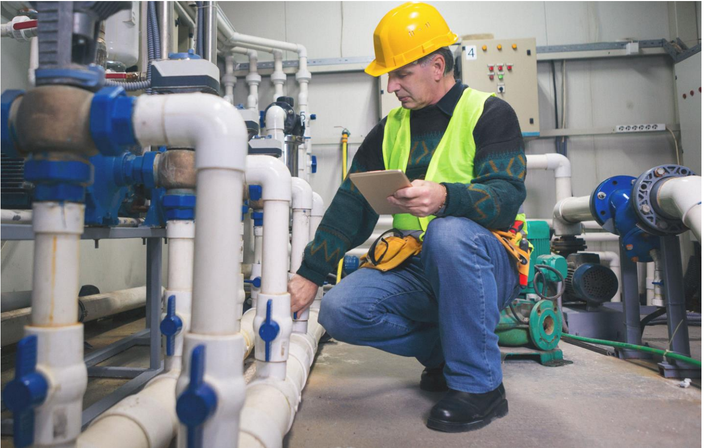
Figure 11: Regular maintenance can reduce the risk of pollution by preventing spills and leaks before they happen.
